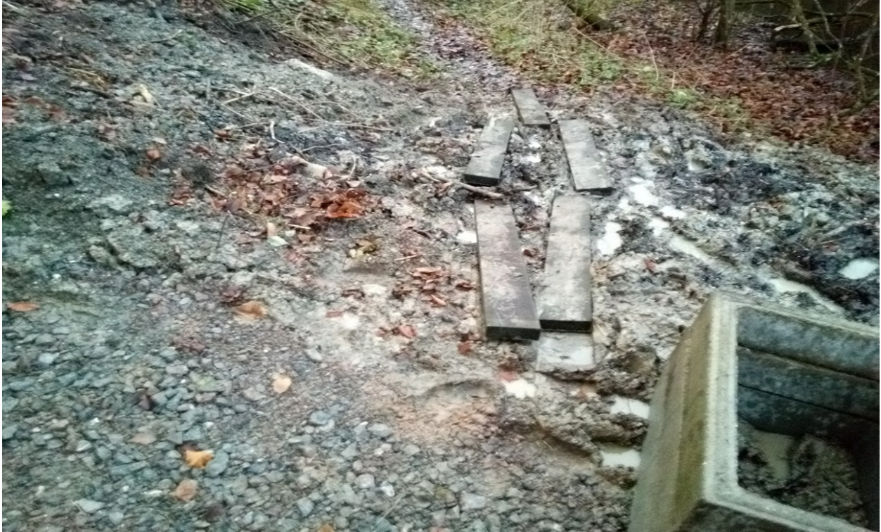
Photo 5a Mud dumped on PROW 7 Dec 2018
